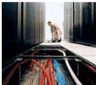
Fig. 79 raised access flooring
