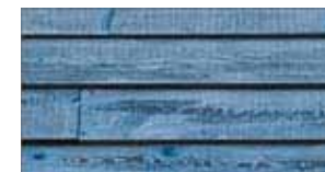
Fig. 21 unfinished wood siding
