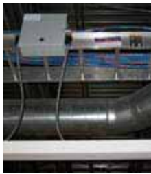
Fig. 50 electrical and telecom raceways
