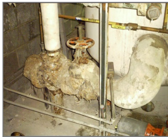
Asbestos pipe fittings
