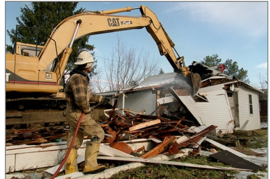
A permit is required to demolish any building, except for residential sheds smaller than 200 square feet
